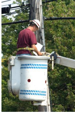
Avoid the electrical wire and report it
